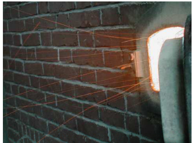
Fig. 1. Sparks and smoke spurting from the furnace as a phenomenon of “puff”.
